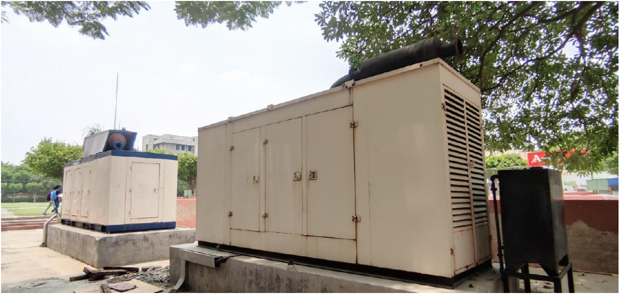
Photo: Generator Facility
