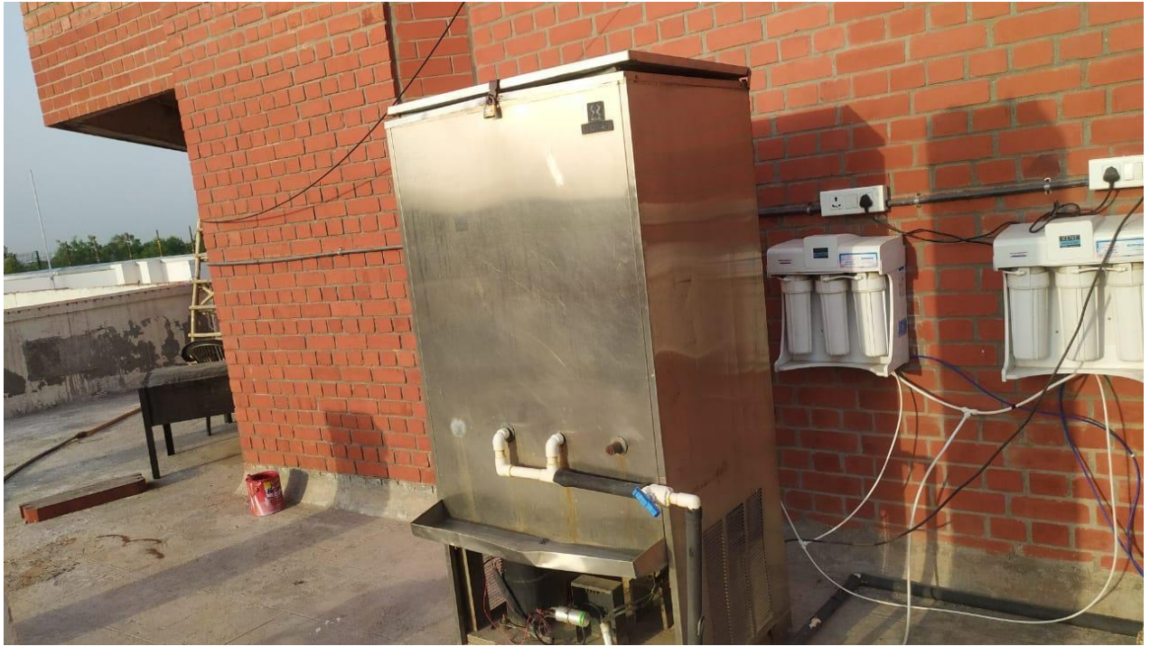
Photo: RO and Water Cooler
